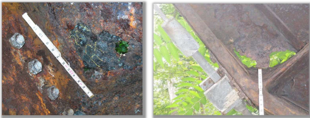
Figure 2. Corroded joint with bolts. Corroded joint with various fasteners.
