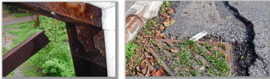
Figure 1. Detached structural joint. Degraded concrete and pavement. Blocked drainage.
