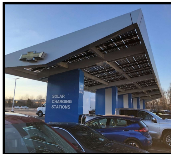
Figure 7. Chevy solar carport with EV charging.
